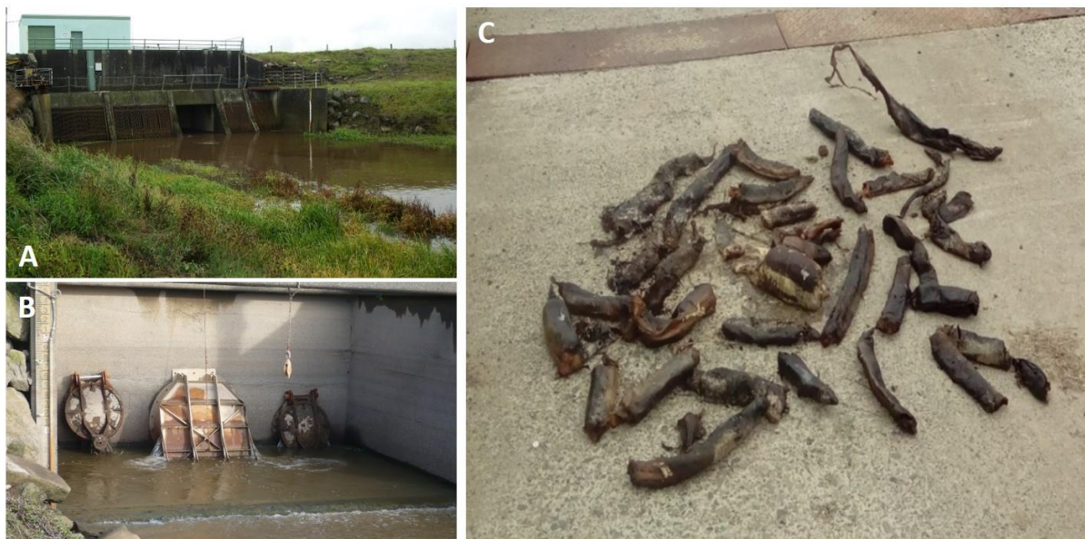
Figure 15: Examples from the Hikurangi Swamp Scheme. (A) A pump station inlet; (B) Flood gates on a pump station outlet; and (C) Some of the tuna killed by one of the Hikurangi pump stations during a flood event in March 2017. (Photos: Jacques Boubée, Alan Halliday). For more information about this particular tuna mortality event, see https://www.maoritelevision.com/news/regional/whangarei-water-turbines-kill-eel-numbers .
