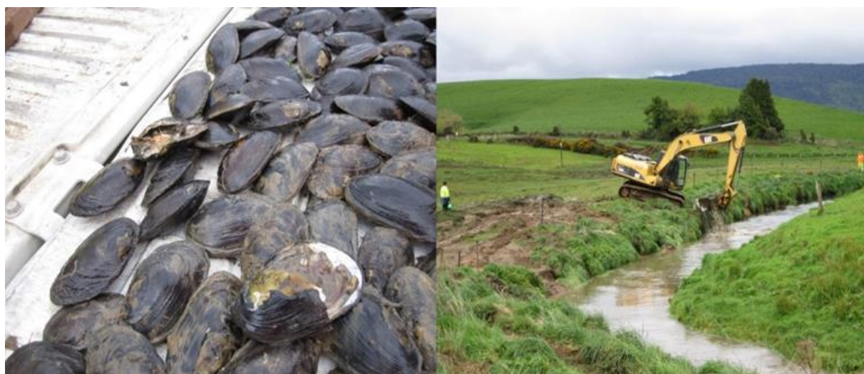
Figure 7: Drain clearing activities in a Murihiku catchment impacting waikākahi (freshwater mussel) populations. (Photos: Jane Kitson). During this incident, in just over 500 m of stream drain clearing, over 200 waikākahi between 65–110 mm were removed from this tributary, which was also close to a nohoanga and mātaihai reserve (J. Kitson, unpub. data.).
